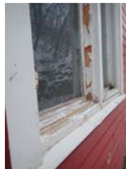
Malings avflassing. Vindu mangler glass
