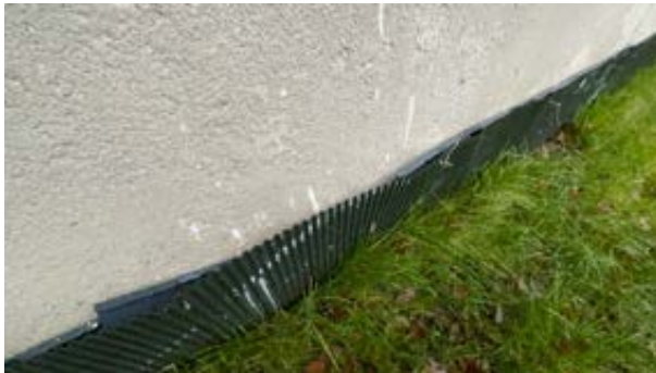
Fuktsikring mangler klemlist
